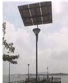
Location: Singapore Solar module: Mitsubishi Electric Client: National Parks Board Application: Jetty Lighting
